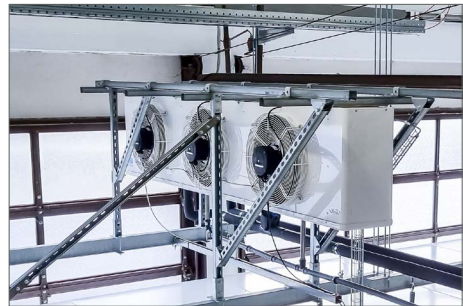
Machine room conditioning
