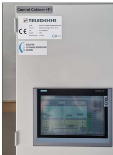
Operating panel with deadman switch
