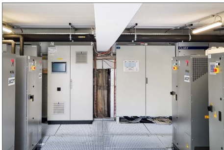
Switch cabinet with S7 controller
